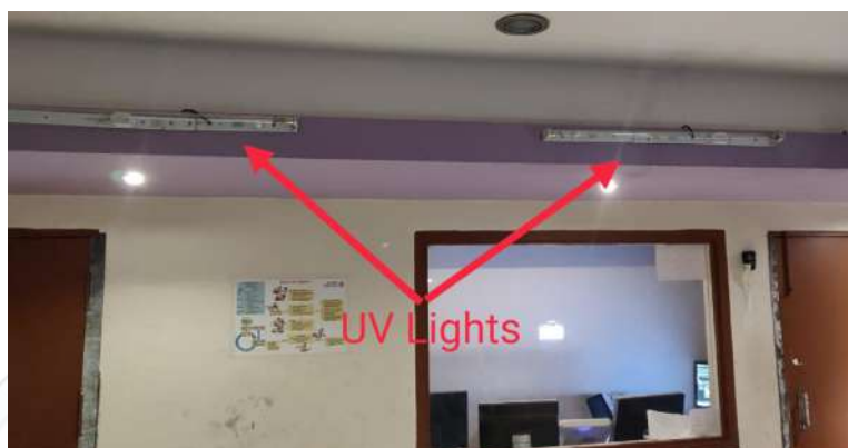
Figure 6: CT room with installed UV lights
